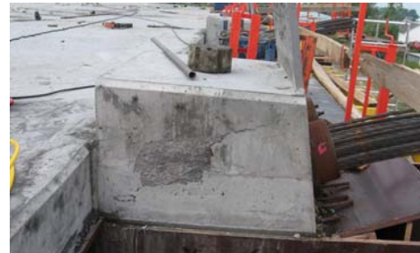
Fig. 3. Damaged cantilever no. 4 after prestressing
