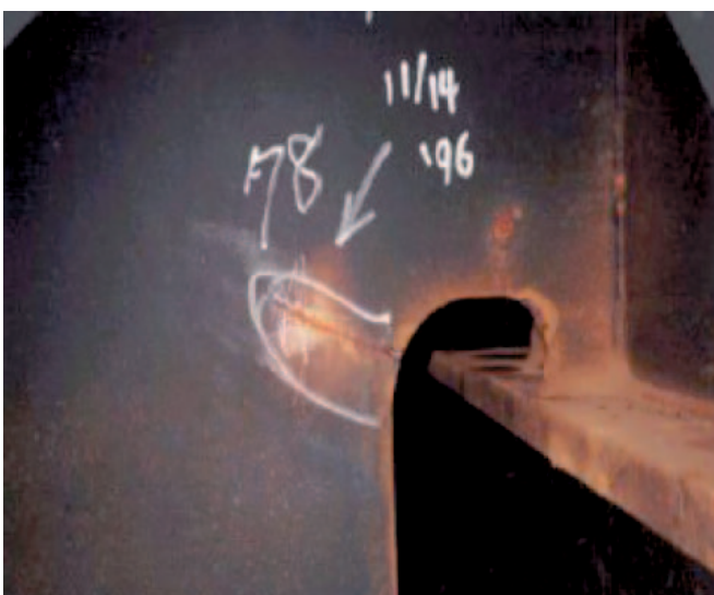
Fig. 4. Example of fatigue crack in base plate of ship structure detail [5]
