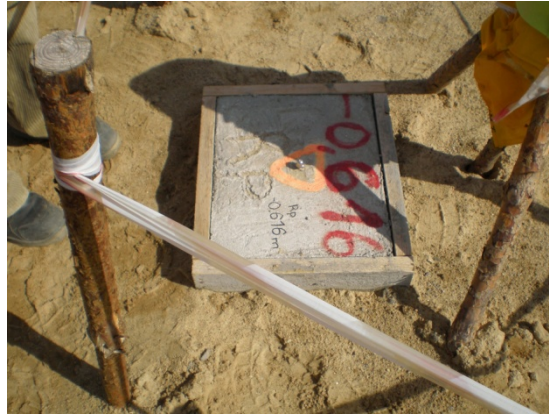
Fig. 10. The central geodetic mark - located in the middle of the stadium plate.
