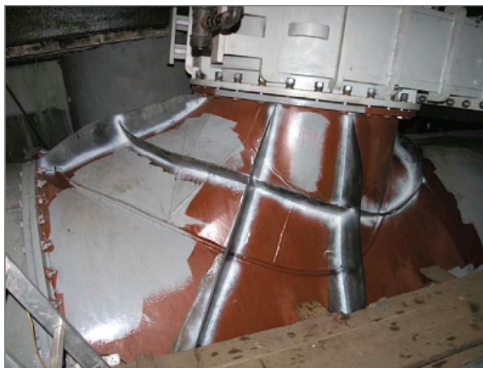
Fig. 19. Bracing webs with reinforcement ring on the inlet pipe. Source: prepared by the authors
