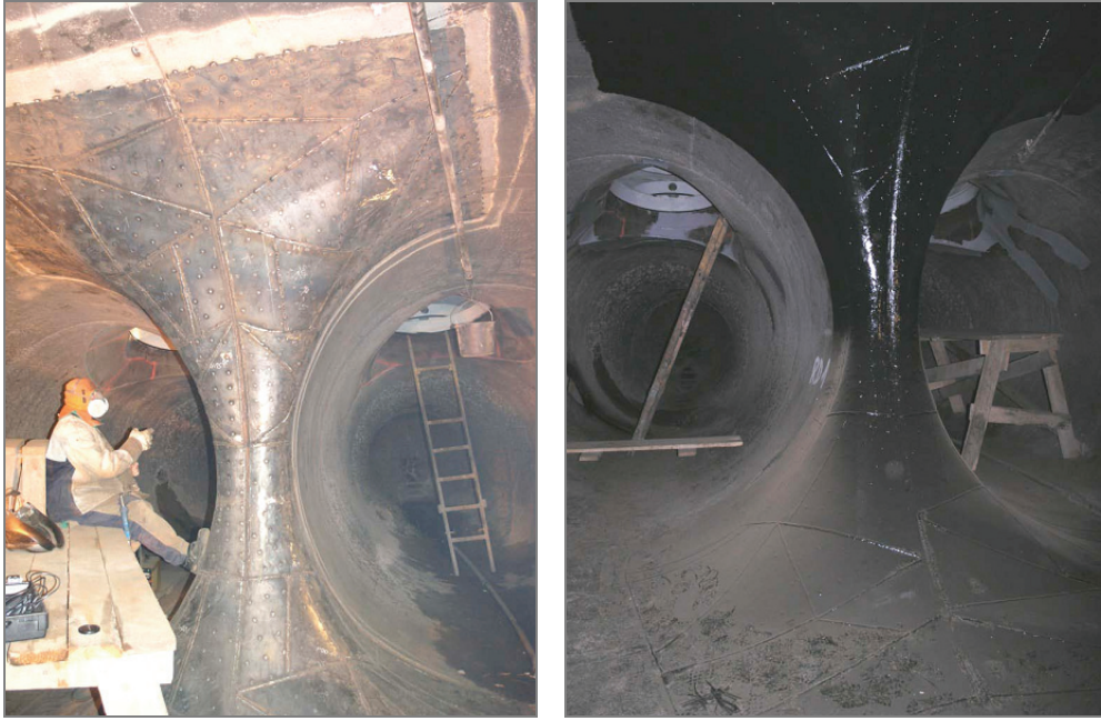
Fig. 17. Structure welding of the reinforcement components to the coating of the pipeline branch and the completed painted plating of the pipeline branch.
