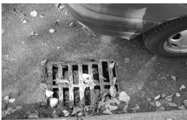
Fig. 1. Fallen withered Oak leaves blocking rain water discharge cesspits found at the side of roads (taken by researcher Nov. 2012).
