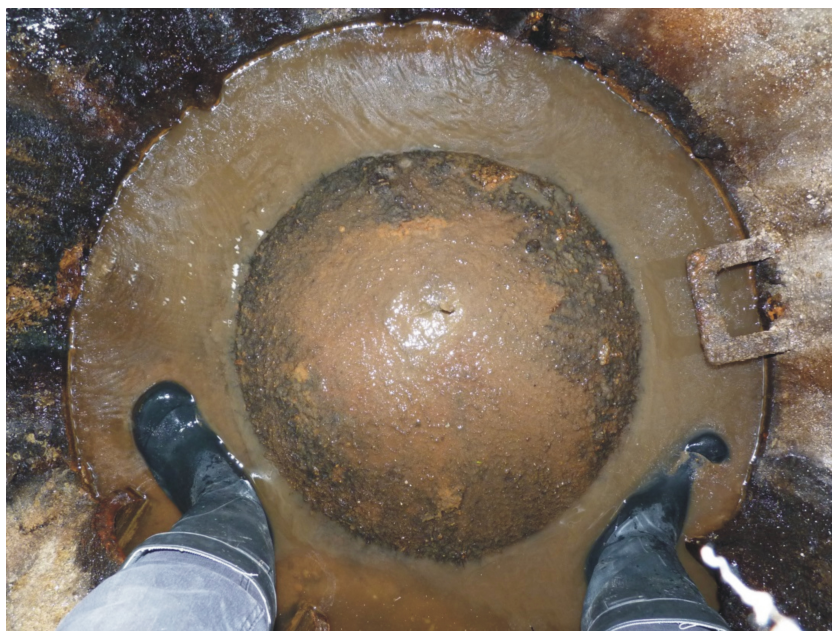
Fig. 5. A bulge caused by groundwater pressure in geotextile at the bottom of a well
