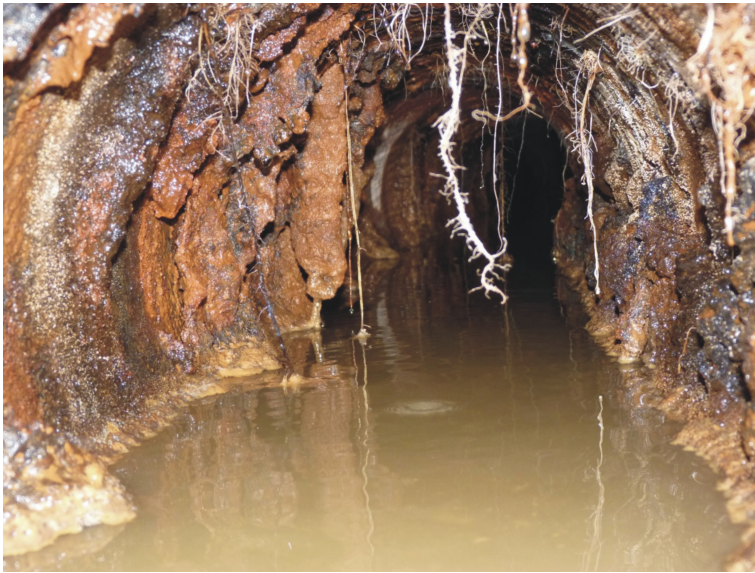
Fig. 4. Ferruginous substance in a pipe
