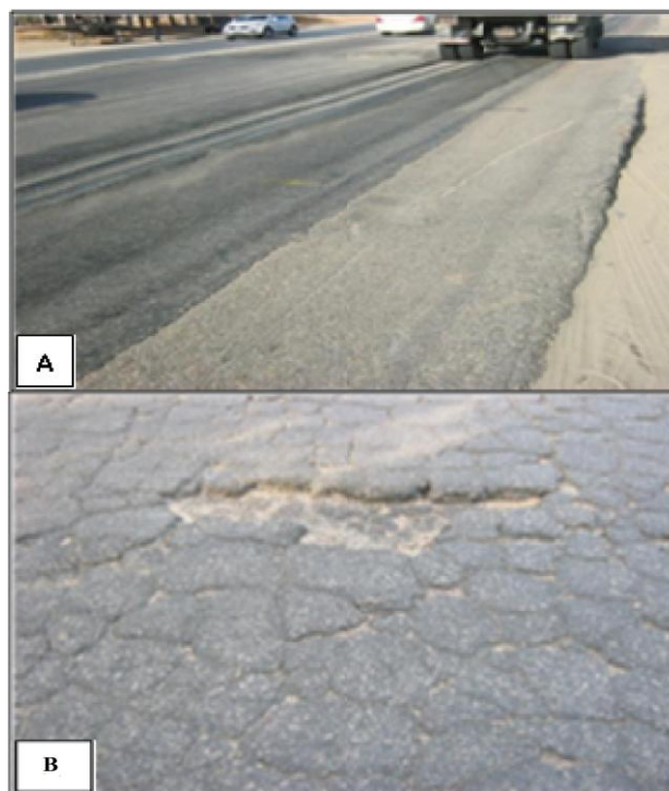
Fig. 2. (A) Rutting; (B) Fatigue cracking [16].
