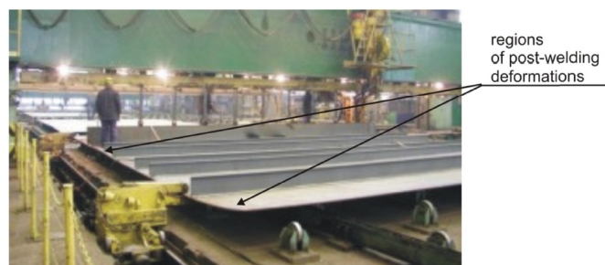
Fig. 1. Welding deformations of a plate section
