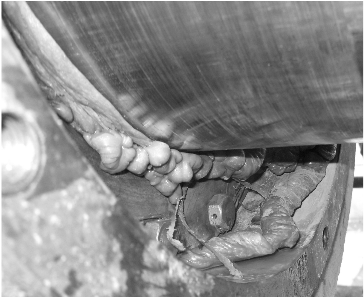
Fig. 1. Melted polymer – the result of an overheated stern tube bearing caused by a cooling system breakdown; shaft diameter 350 mm.
