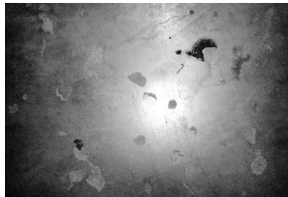
Fot. 2. Uszkodzona posadzka parkingowa na skutek korozji [Fot. Autorki] Photo 2. Damaged floor parking due to corrosion [Phot. Authors]
