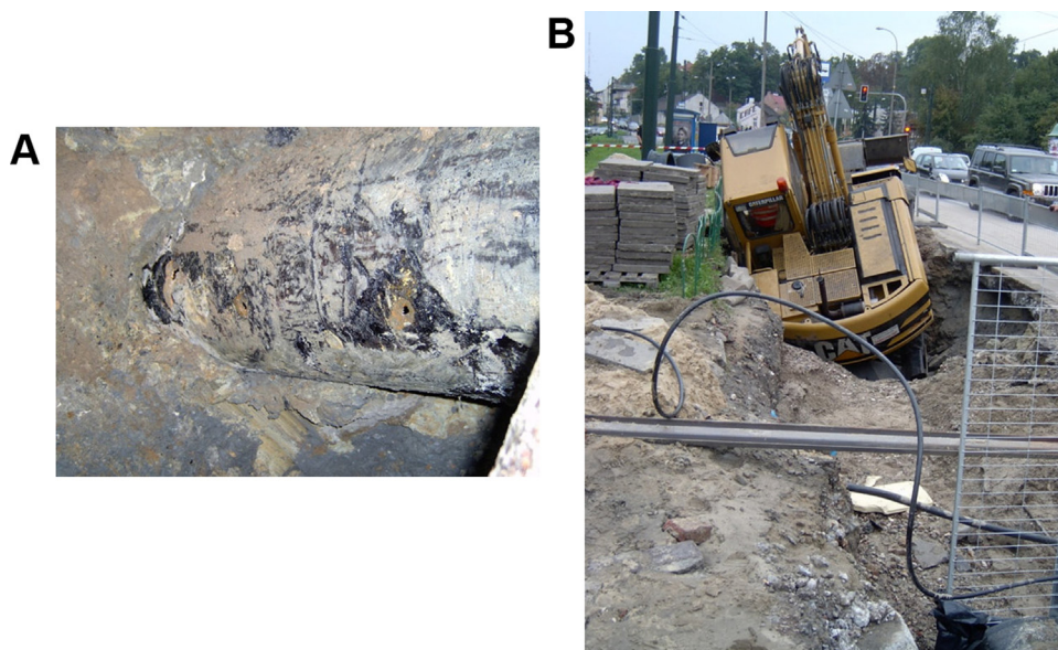
Fig. 1. Local corrosion of a DN300 pipeline.
