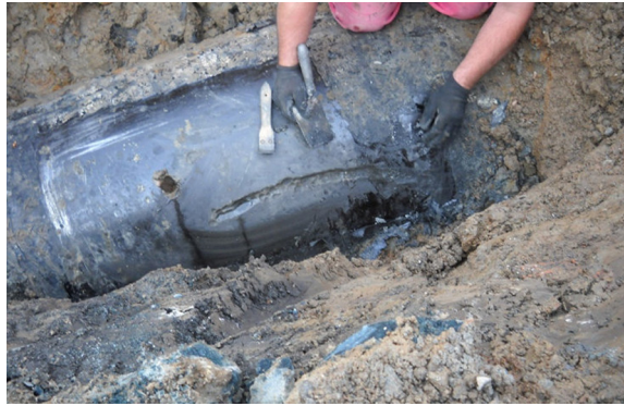
Fig. 1. View of pipeline corrosion failure.
