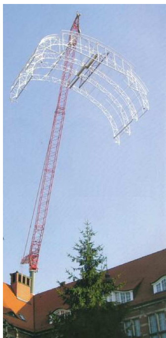
Fig. 19. Transferring glazed roof framework from the assembly site onto the Hevelius Courtyard (CYWIŃSKI, 2012).
