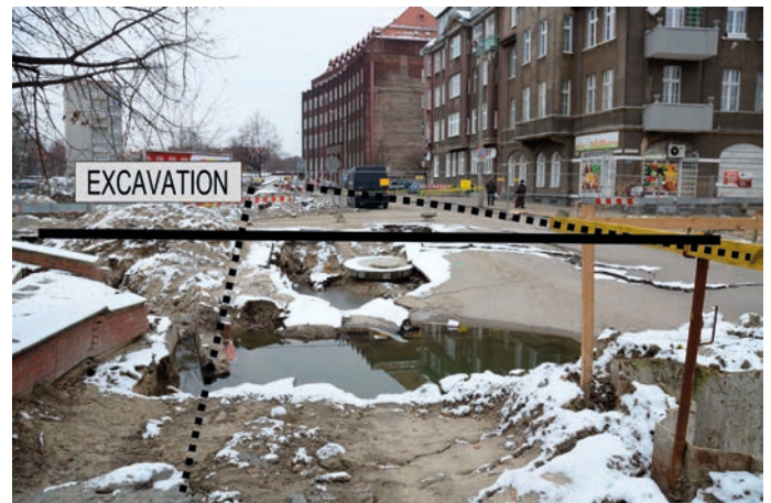
Figure 12. General view of Gdańsk 2013 real-life case of a pipe failure in the vicinity of an unsecured excavation that inspired this study Dotted lines indicate road edges while solid line indicates the axis of the pipeline
