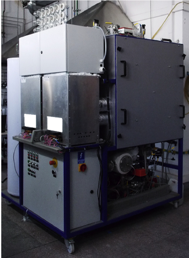
Fig. 30 – Micro-combined heat and power unit with SOFC, design and constructed in the Institute of Power Engineering.
