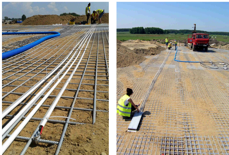
Fig. 7. Long base extensometers for measuring elongation of the steel grid
