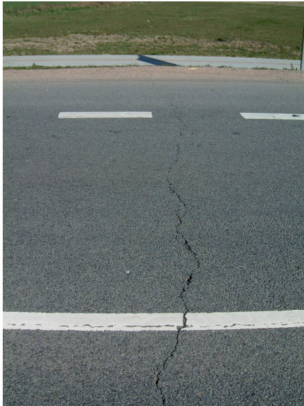
Figure 1. Transverse crack in the national road No. 7.
