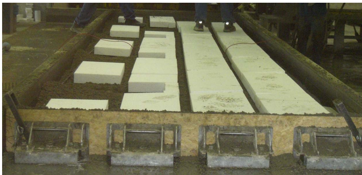
Figure 3. The reinforced wall component (the first improved type) during the concreting process
