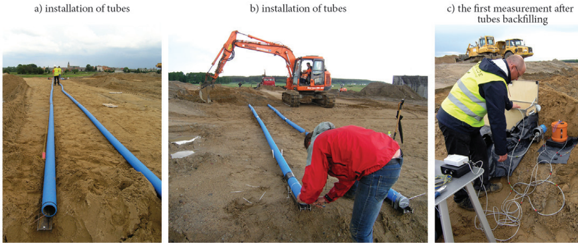
Fig. 8. Embankment settlement measurement by hydrostatic levelling
