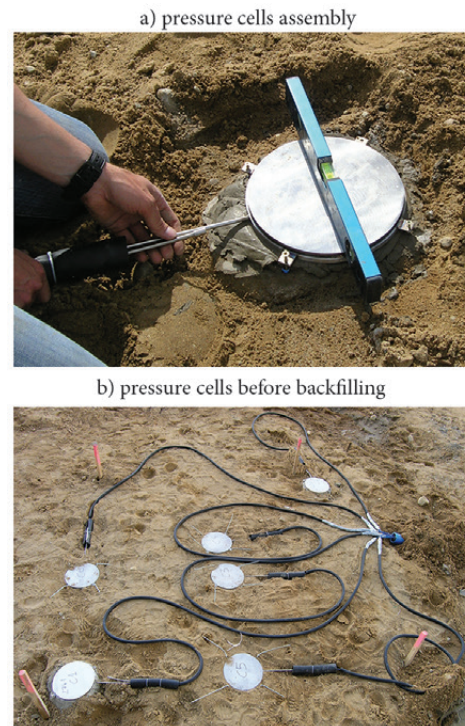
Fig. 5. Vibrating wire load cells measurement points
