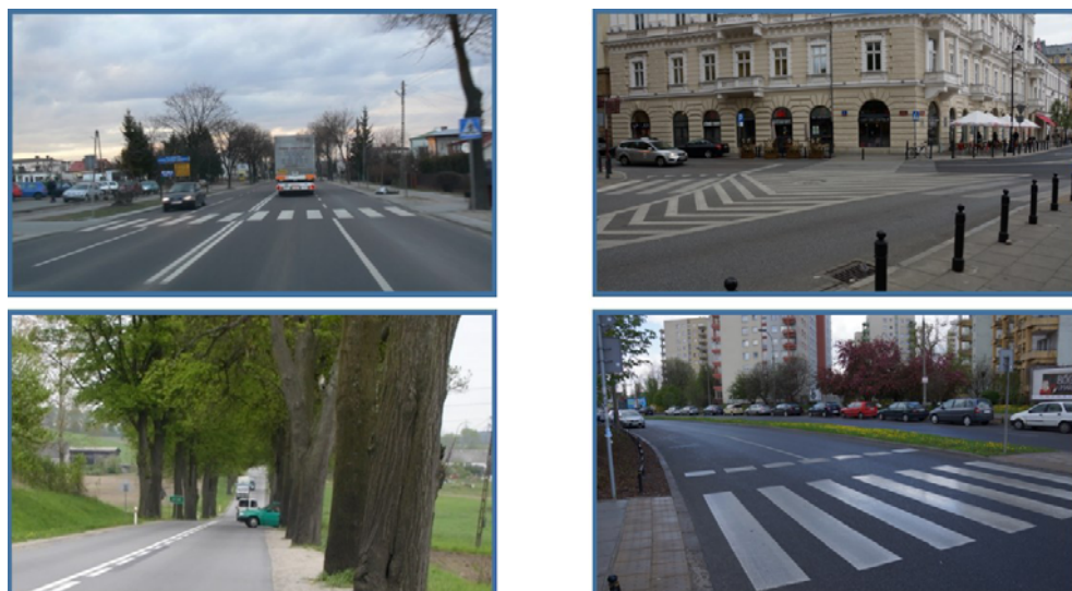
Fig. 3 Examples of road defects.
