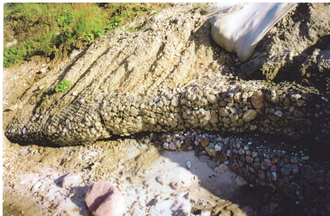
Fig. 3. Gabions composing the seawall in the region of "Bałtyk", damaged in 1998 (photo courtesy of W. Subotowicz)
