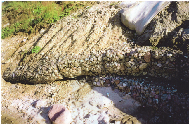
Fig. 3. Gabions composing the seawall in the region of "Bałtyk", damaged in 1998 (photo courtesy of W. Subotowicz)
