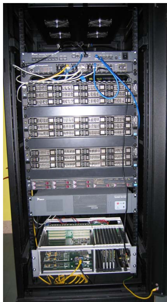
Figure 2. From the top: URC for OP, switch, Archive Servers (AS), voice recorder, telephone server.
