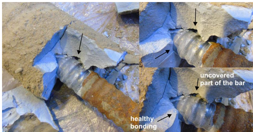
Figure 7.31 Damaged anchor: uncovered part of the bar and healthy connection at the anchorage place
