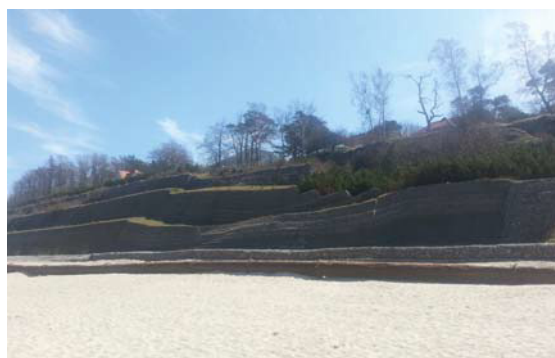
Fig. 3. Deformations of the cliff protection structure made of reinforced ground and gabions (2014) [8]
