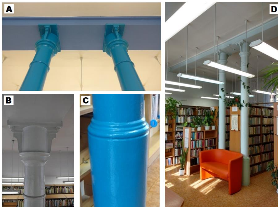
Fig. 3. Cast iron columns in the building of the former financial office in Kwidzyn: A - view of the beam's double support, B – detail of the column capital, C - base detail, D - general view.
