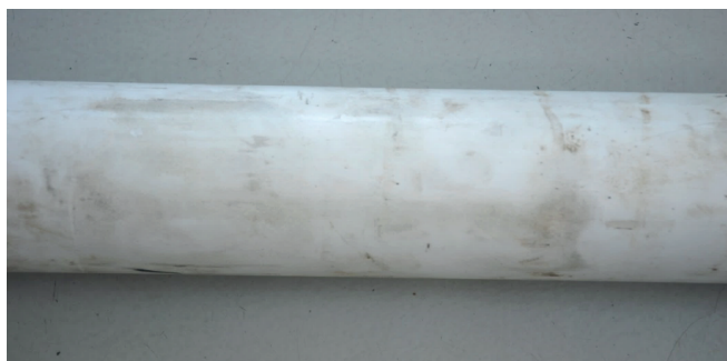
Fig.12. Condition of CTP pipe protection layer after tests – no outer layer damages
