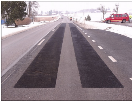
Figure 13: Swedish full scale test tracks in Sjögestad in February 2016, i.e. 1,5 years and two winters after construction. The Sjögestad II surface with the PERS prefab panels (applied only in both wheel tracks) can be seen on the foreground. Note some scars by the snowplough and some raveling. The slightly lighter coloured PERS surface in the background the original in situ constructed PERS test track (Sjögestad I)
