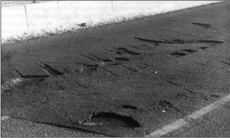
Figure 3: Damages to PERS by snow plough ending experiment in Oslo [4]
