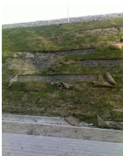
Fig. 2. Negative impact of the incorrect drainage on the condition of embankment slope (registered in March 2017)
