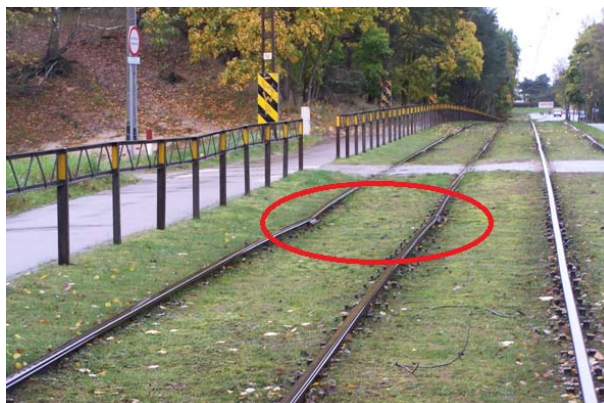
Fig. 3. Displacements of the sleepers in the track
