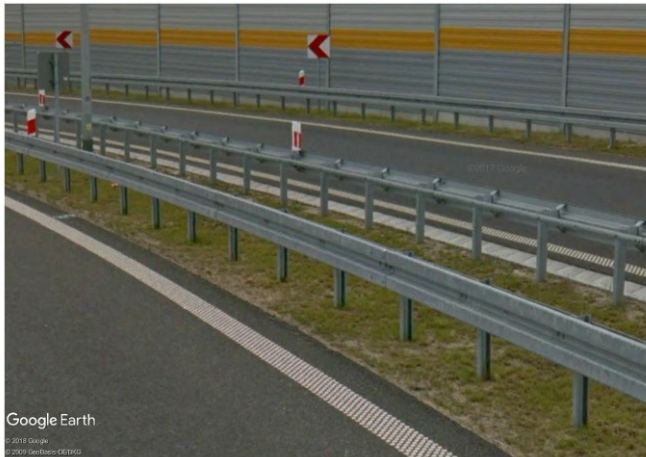
Fig. 1 N2/W4/A steel road safety barrier on A1 highway in Poland, credits: Google Earth.
