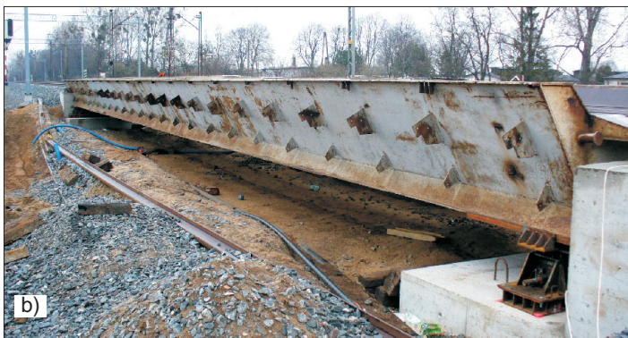
Fig. 1. KO30 bridge span: a) the cross-section scheme, b) the view of the span in service - track No. 2 PKP PLK
