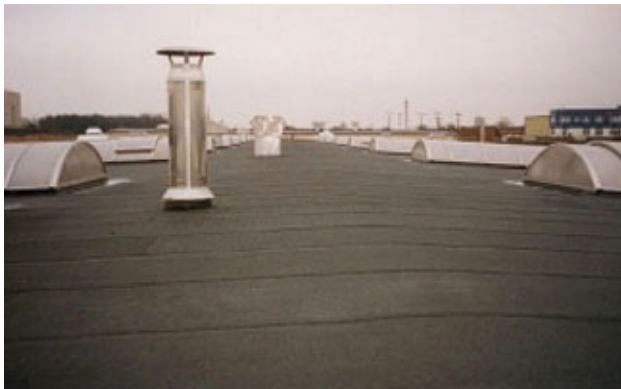
Figure 1: The view of the roof area with an area of 1000m 2 selected for conducting this analysis.
