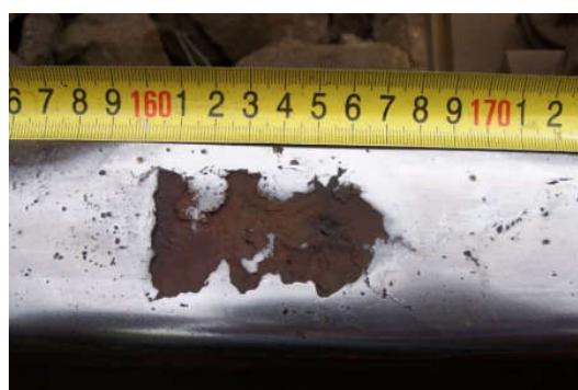
Fig. 3. Measurement of defects.
