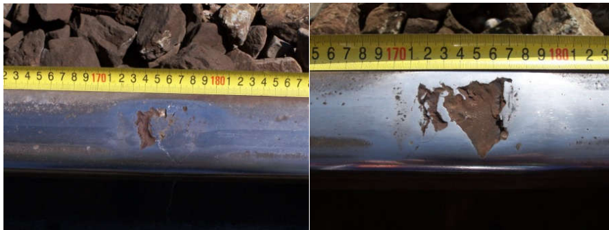
Fig. 4. Development of defect in the rail over a period of 15 months of rail exploitation.
