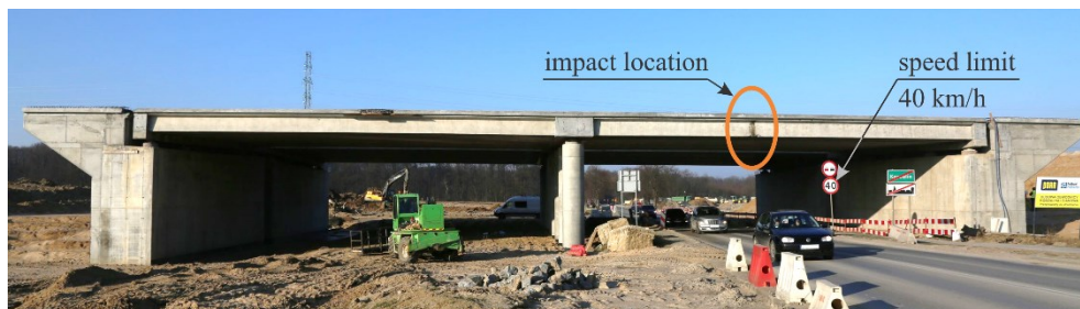
Fig. 1. Overall view of the bridge. The location of the impact is marked orange.
