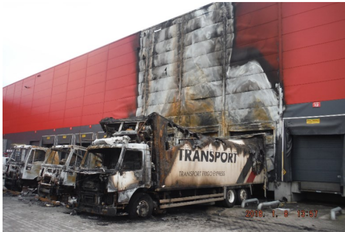
Fig. 1. View of fire damaged lorries and warehouse façade.
