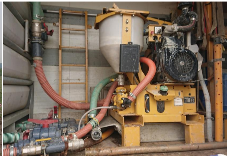
Figure 6. The system for preparation of drilling fluid.
