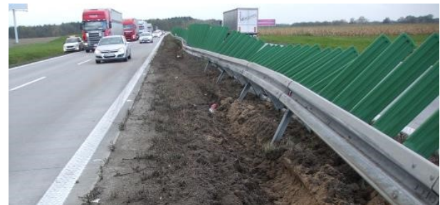
Fig. 6. Photographic documentation of road accidents /source: General Directorate of National Roads and Motorways/
