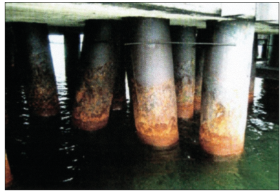
Fig. 6. Sea corrosion of piles [10]
