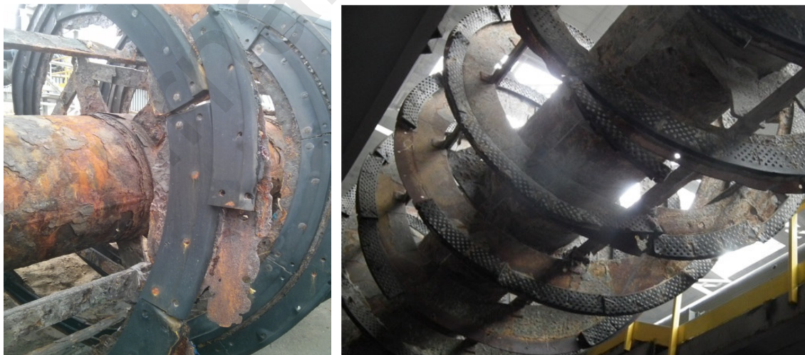
Photo 4÷5. Classifier's spirals degraded due to corrosion.
