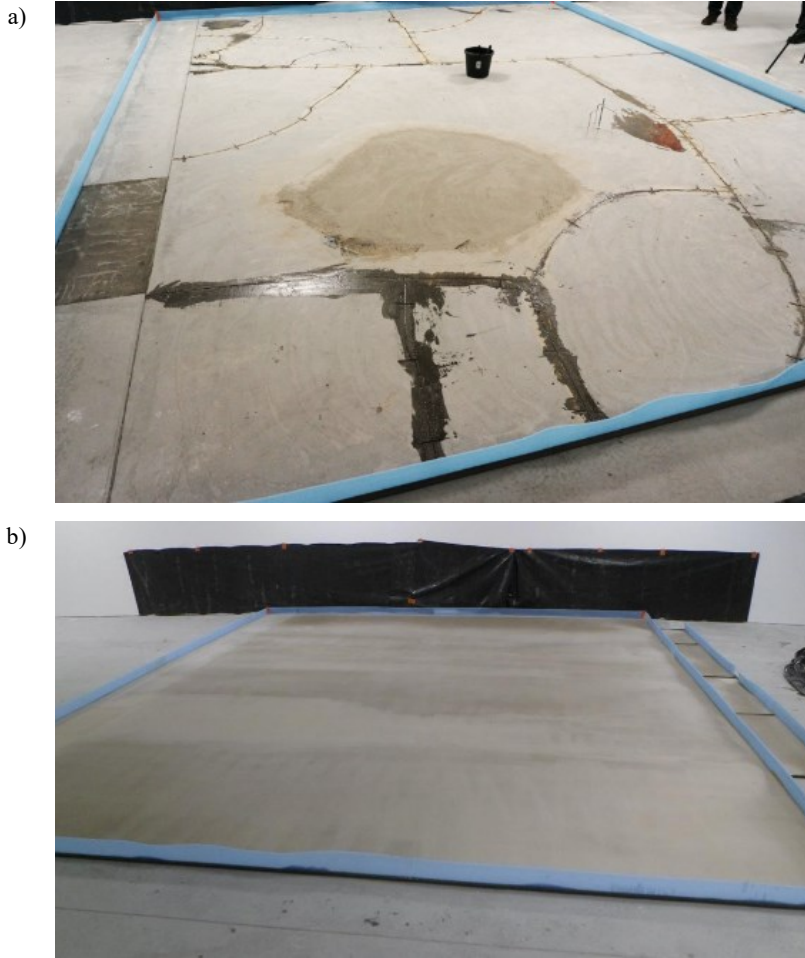
Fig. 13. Repair method: a) view after stitching and injection of the cracks, b) finished top layer.
