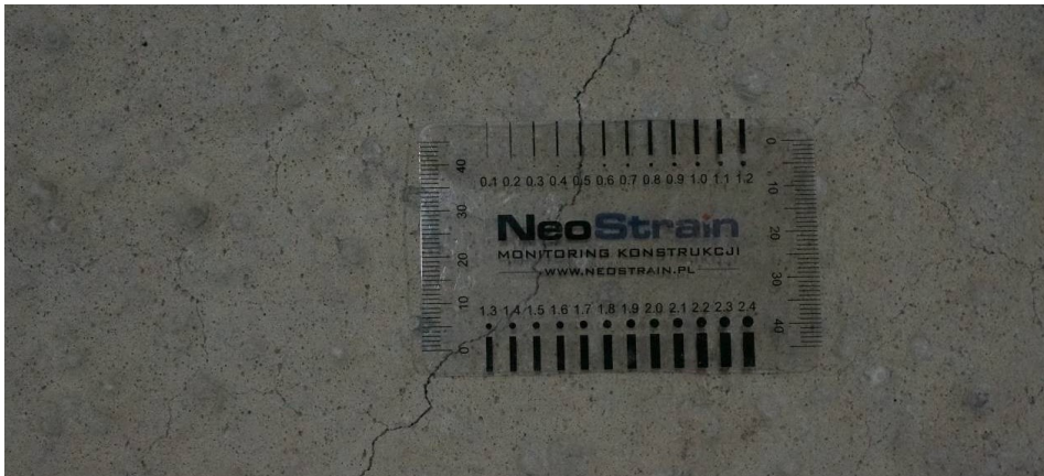
Fig. 10. Measurement of the cracks in sample no. 4.
