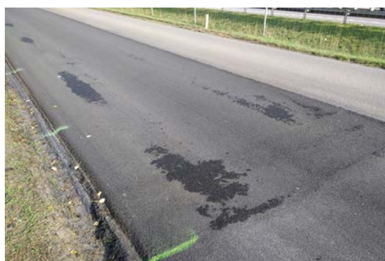
Figure 22. Transvers mark caused by paver stop on the Galaktyczna street trial section.
