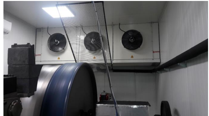
Fig.7. Thermostatic chamber used in the tire testing laboratory of the Gdańsk University of Technology (own material)
