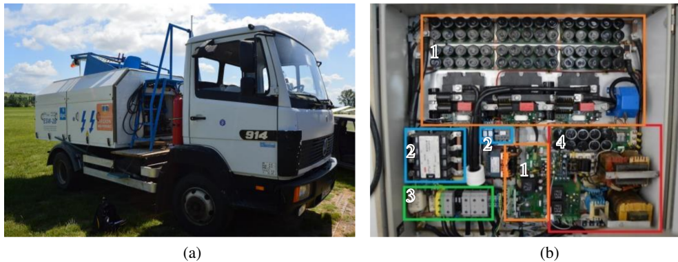
Fig. 1. View of the studied launcher Electronic circuits: (a) Mercedes-Benz model 914; (b) all power electronic components of the launcher (1. inverter with control driver, 2. contractors and relays, 3. fuses, 4. battery charger with driver)
