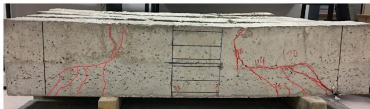
Fig.11: Beam (B3) at failure
