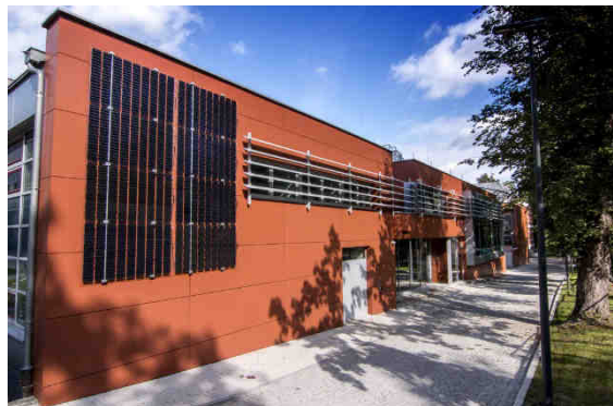
Fig. 4. View of the whole BIPV system on the south-east building facade
