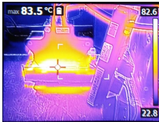
Figure 11. Temperature measurement of the second developed MFT with split windings at power of 45 kW without forced cooling.
