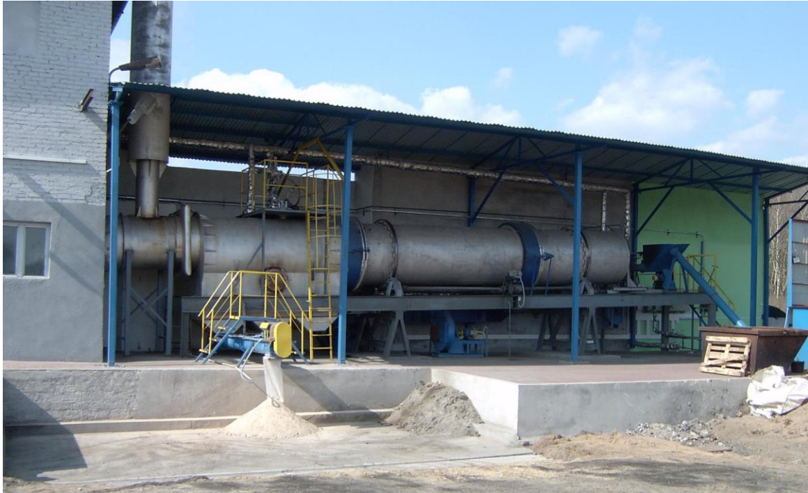
Fig. 2. General view of the installation.
