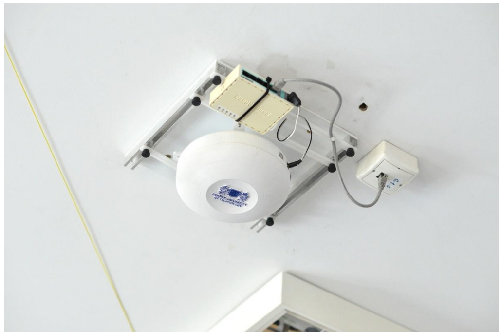
Figure 8. The ESPAR antenna integrated together with the custom-made WSN board installed within a custom-made housing and mounted on the ceiling.
