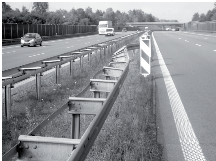
Fig. 1. View of damaged road barrier as a result of vehicle impact, impact angle was approx. 8 degrees (source: GDDKiA)
