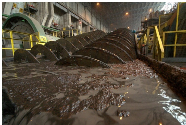
Figure 1. View of a working two-winding classifier.
