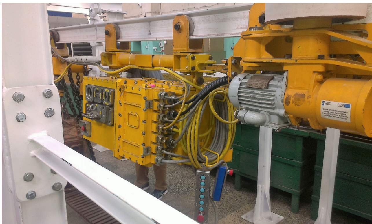
Figure 2. General view of the suspended battery vehicle PCA-1.
